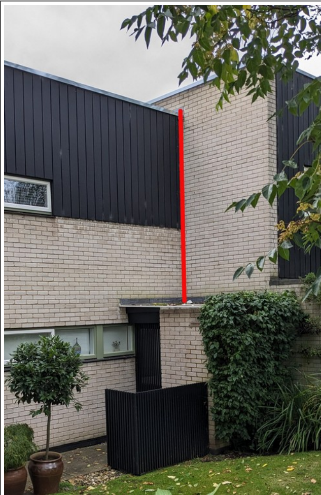
This is most useful for the house on the left as it goes direct to the utility room
